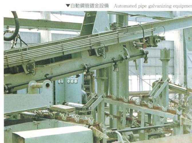
▼自動鋼管鍍金設備 Automated pipe galvanizing equipment
