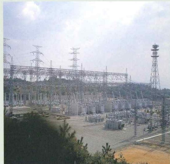
▼発電所屋外鉄構 Steel structures for power stations and substations
