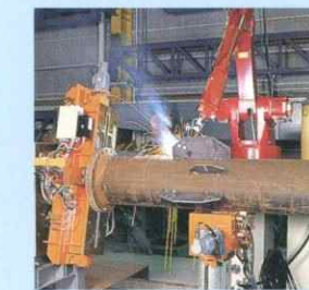
▲主材ロボット溶接装置 Welding robot for tower main post members
