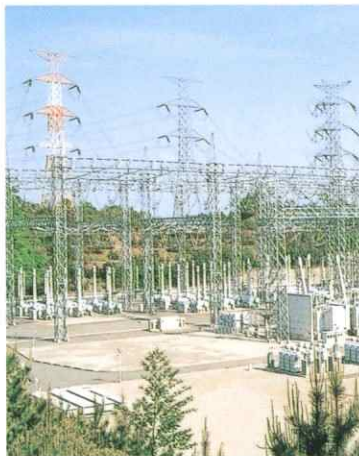
▲関西電力信貴変電所 Steel structures in a substation of The Kansai Electric Power Co., Inc.
