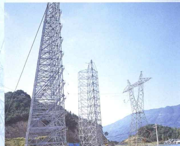
■琴平鉄塔実規模試験場 (14,257㎡) Full scale tower loading test station in Kotohira
