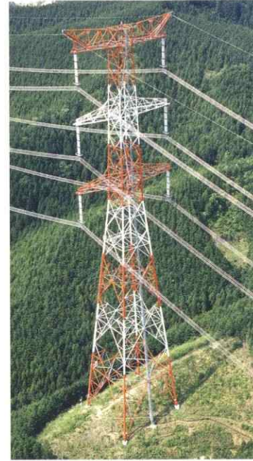
▲東京電力南いわき幹線UHV (1,000 kV) Ultra high voltage (UHV) Minami-Iwaki trunk transmission line tower of The Tokyo Electric Power Company, Inc.
