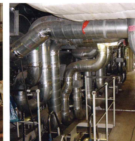
空気調和装置 (Air-Conditioner) 空調機室内スパイラルダクト Air Conditioning Room Spiral Duct (Pre Insulated / Bare)
